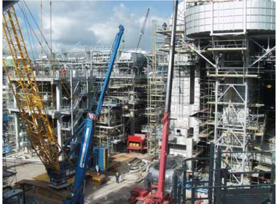
Right. Preemraffs refinery in Lysekil, Sweden. A major project with 3,000 tons of pipes to be installed. The Swedish contractors and plumbing firms couldn't compete with imported labour and piping installations which were done by Thai installers and service contractors. Photo: Anneli Megner.
