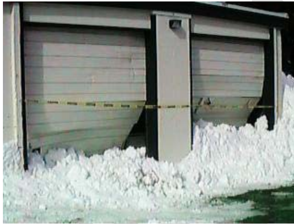
The weight of built up snow can easily damage buildings.
