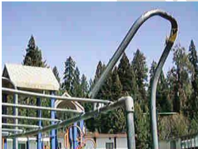
Property damage from excessive snow weight.
