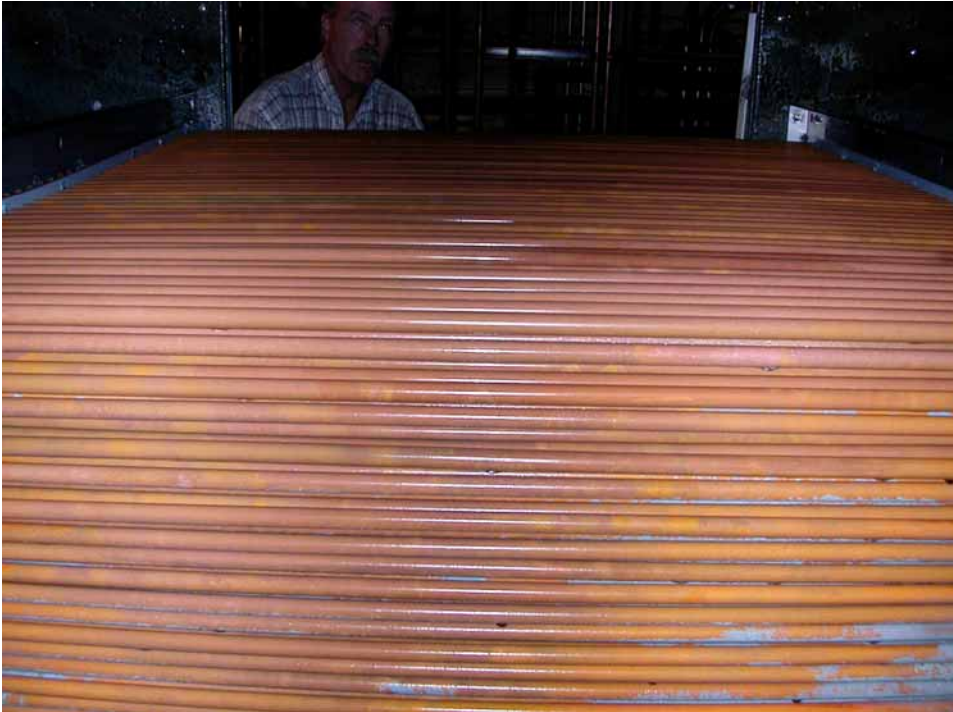
Figure 43 Arcadia cooling system prior to treatment with Scale Viper
