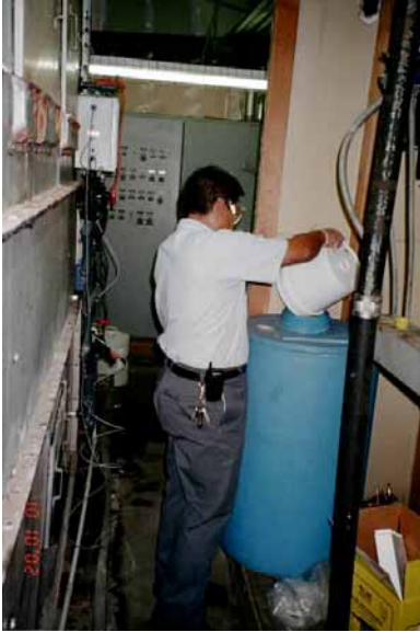
Figure 55: Chemical storage tank at Irvine
