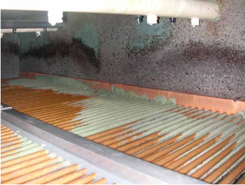
Figure 85: Scale on top of USC tubes in December, 2002
