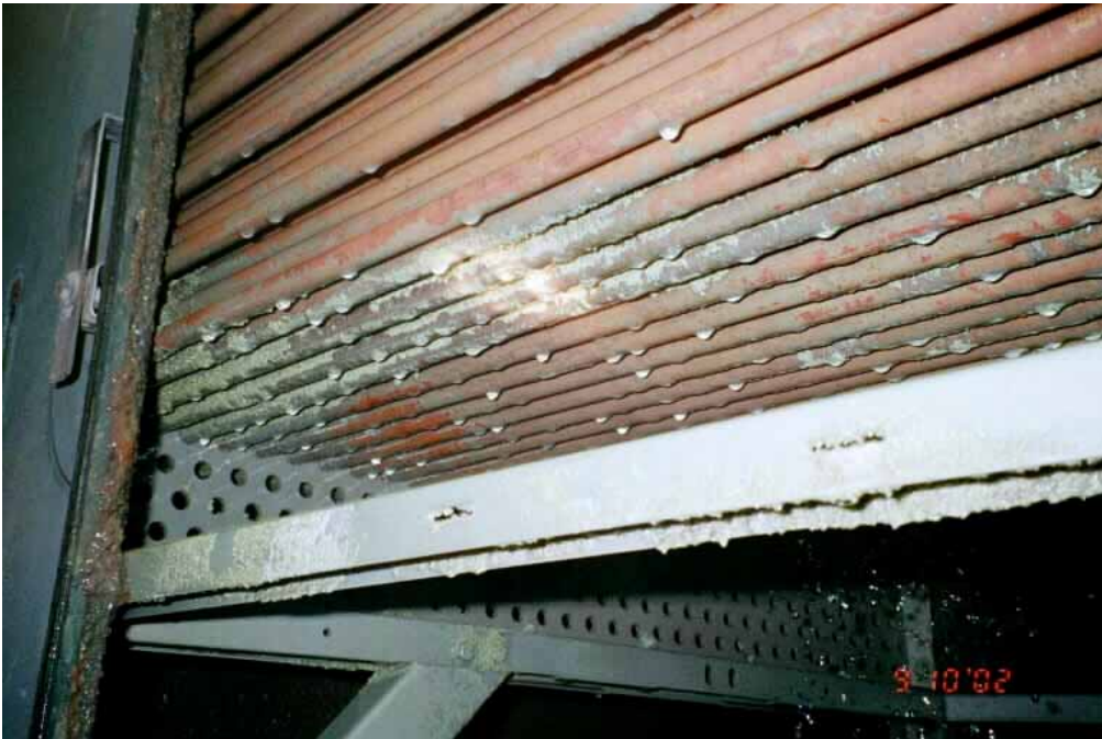
Figure 73: Santa Monica cooling tubes from bottom, Oct. 2002
