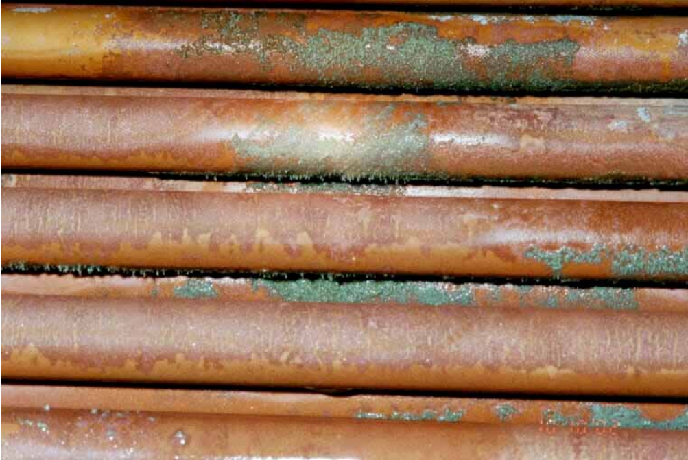
Figure 63: Irvine pipes side-view close-up, October 2002
