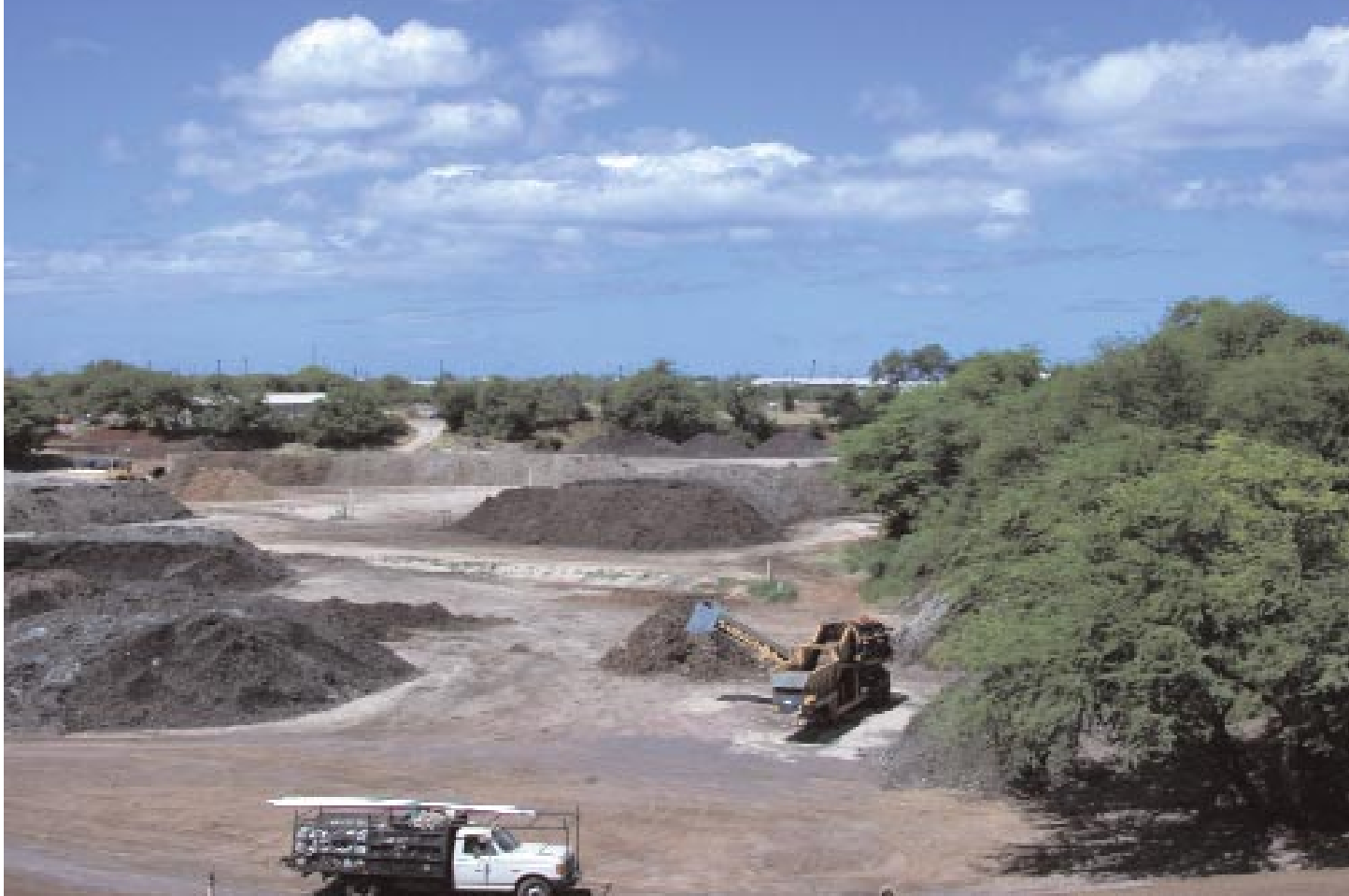
An overview of the NAVFAC Hawaii Biosolids Treatment Facility showing various mixing areas and composting and curing piles. Denise Emsley
