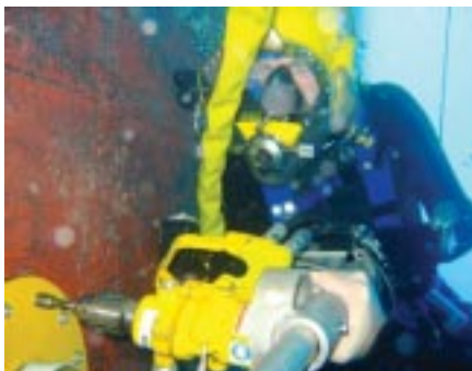
A Navy diver from MDSU 1 installs self tapping screws using an underwater hydraulic impact wrench while installing a hot tap flange on the M/V Tong Cheng. Photo by Navy Diver 1st Class Jason Mette
