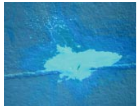
Temporary repairs conducted by the MDSU 1 scuba team. Waterproof epoxy was used to fill the cracks and control the flooding prior to surface supplied diving and pumping operations once the vessel was moved close to shore.
