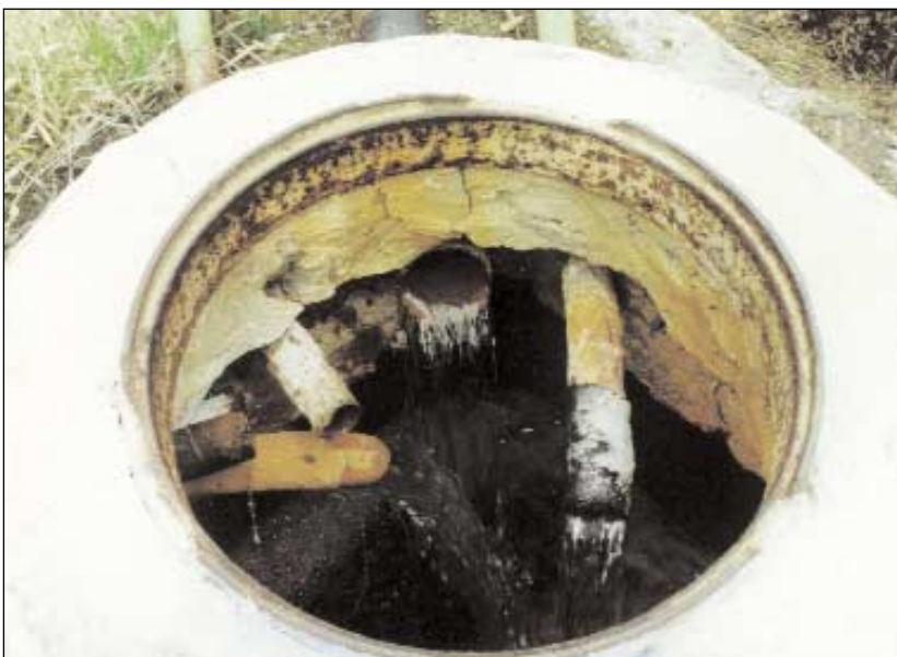
Figure 4 Rusting and disintegrating pipes
