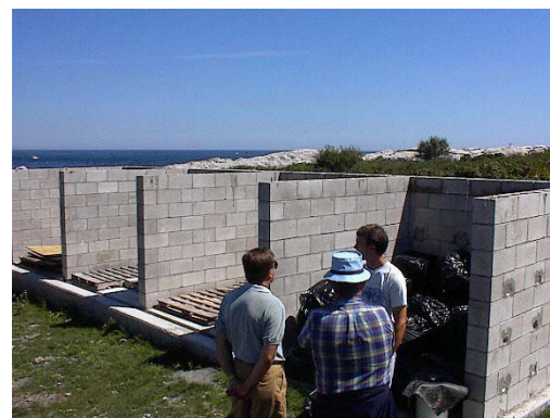
Oceanic Hotel Compost Bunkers
