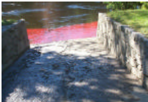
Erosion at a boat ramp
