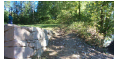
Another example of erosion
