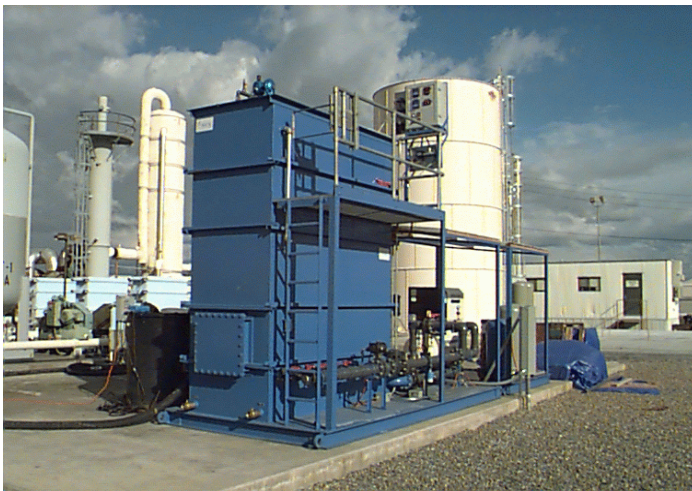
Bioreactor installed on demonstration test pad at the base's Groundwater Treatment Plant. All utilities and service connections are provided by the Test Site.
