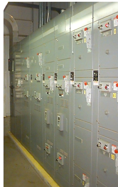
Figure 3: Variable Frequency Drives
