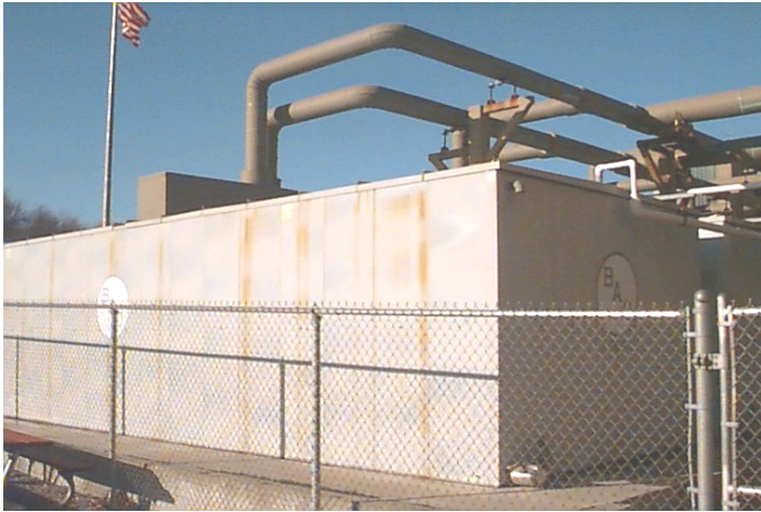
Figure 3: Building 12 Ice Storage System
