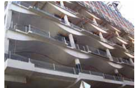
Figure 15. CH 2 during construction photo of high thermal mass wavy ceilings, City of Melbourne. (6 Star Green Star - Office Design v1)
