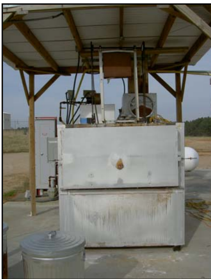
Figures 4 a & b. Gasifier located at NCSU APWMC WPF.
