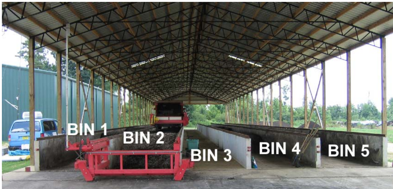
Figure 4.3 Cross-sectional view of composting barn showing 5 bins for holding composting material. Mechanical mixer is mounted on railing above Bin 2.
