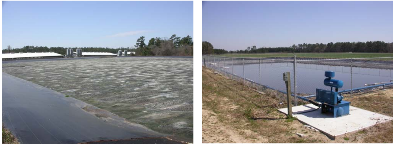
Figure 4. Images of the Permeable Cover System (PCS) – Permeable covered lagoon and aerobic digester.
