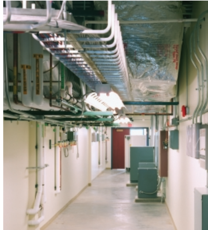
Separated utility corridor provides minimal disruption for maintenance of mechanical equipment, electrical, and plumbing for laboratories.
