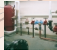
Pressurized holding tank for the rain water.
