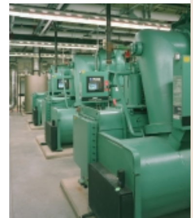
Small water-cooled chillers.
