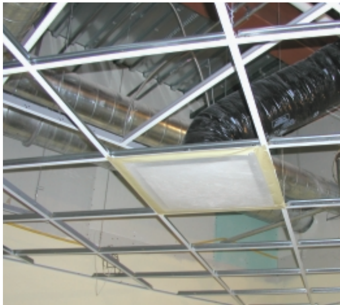
During construction, the HVAC system and duct work were sealed on a daily basis to prevent infiltration of any dust, chemicals, or odors due to construction.
