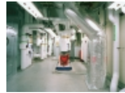
White pipes on right carry rain water drained from the roof.
