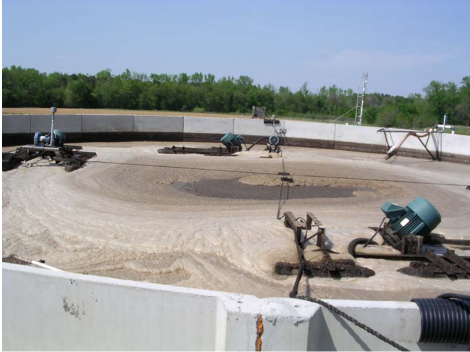
SBR reactor under normal operating conditions
