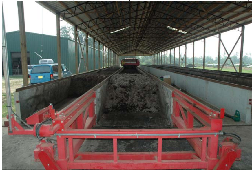
Figure 6: Front of compost bin #2 showing railing system and dock (foreground) used to move the mechanical mixer along the bin and across bins.
