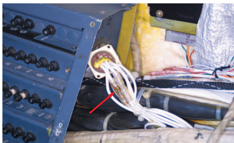
Figure 3. Close-Up Of Butt Splice Terminations in a Circuit Breaker Panel.
