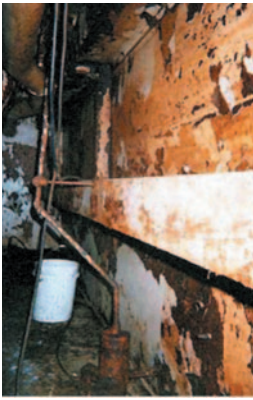
Figure 1. Interior of a Ballast Tank on a Navy Ship[4].
