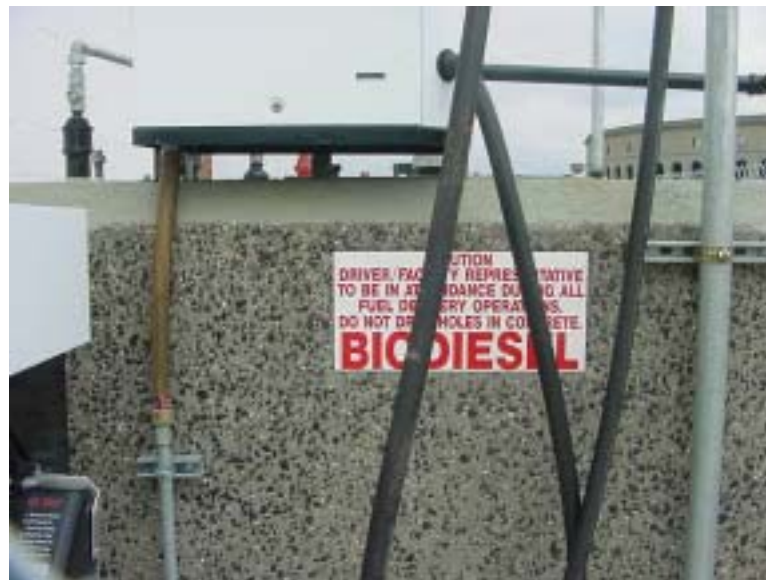
Explosion Proof Wiring
