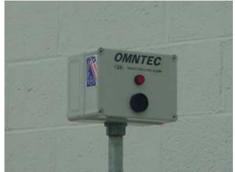
High Level Alarm
