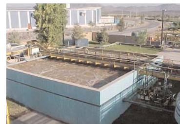
Aeration tank of the biological treatment system for Industrial wastewater
