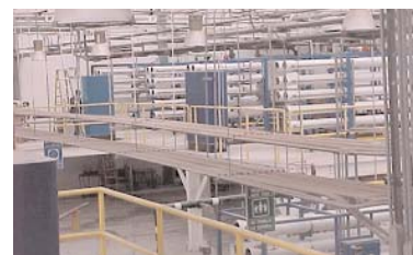
Reverse osmosis units of the brine-recovery system and the well water treatment system
