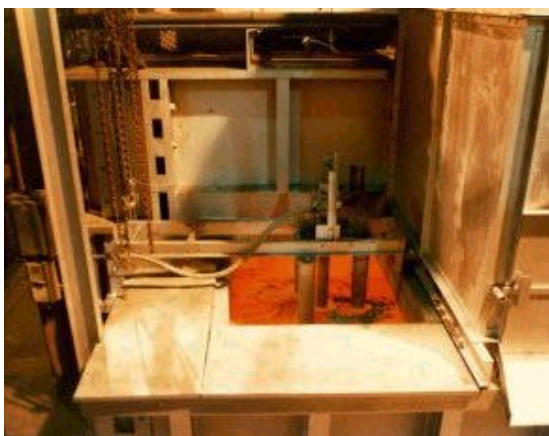
Figure 17 Mechanical Pumping System (Vortexer type courtesy G+P Inc.)
