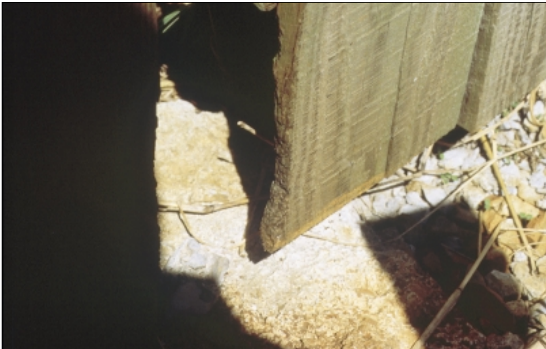
Figure 5 Holes in stores should be repaired to exclude rodents. Photo courtesy of Bell Laboratories, Inc
