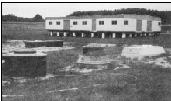
Training center classroom under renovation; aerobic treatment unit and peat biofilter demonstrations in foreground.
