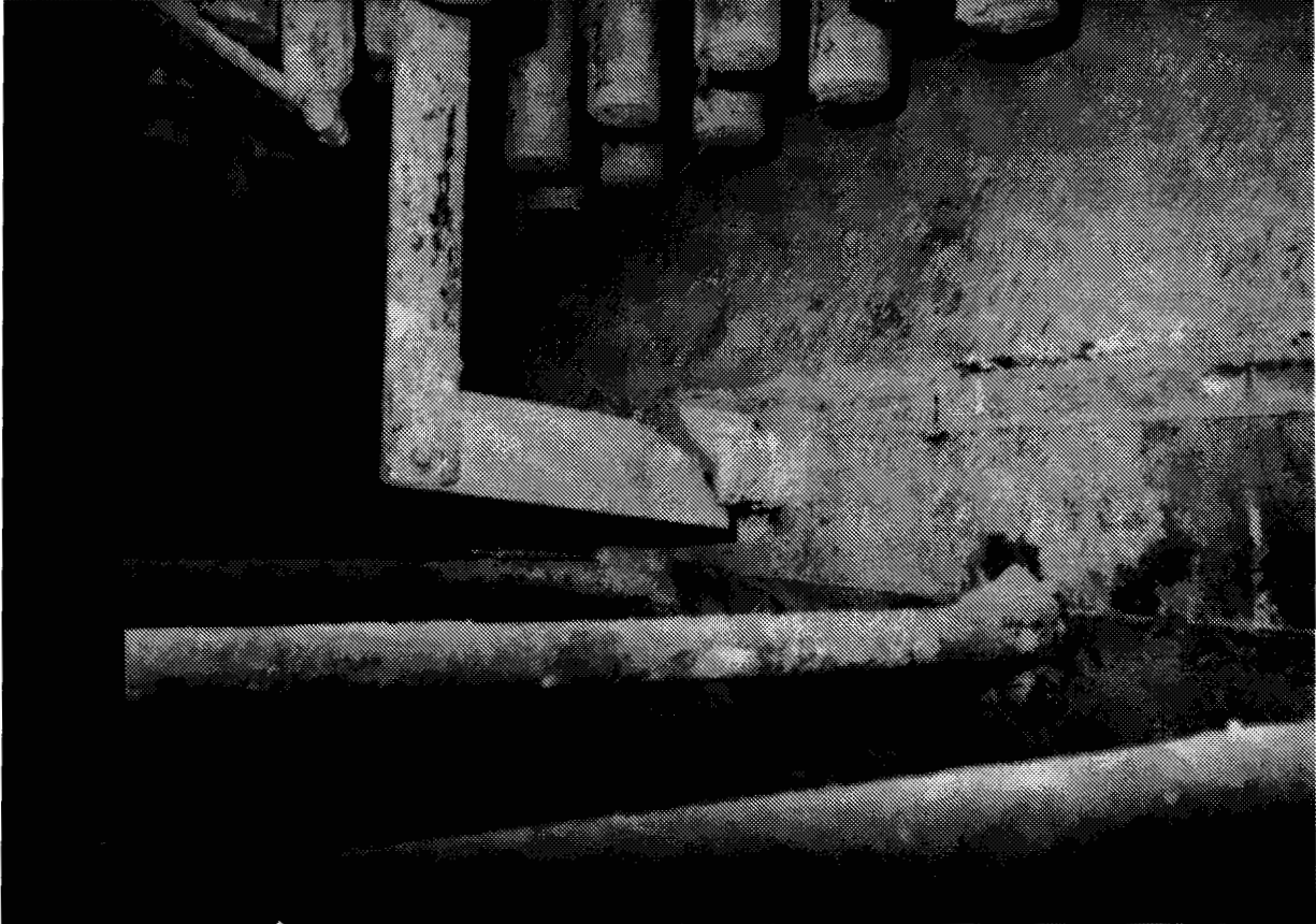
Figure 6-23. Photograph of broken plate stabilizing bracket.
