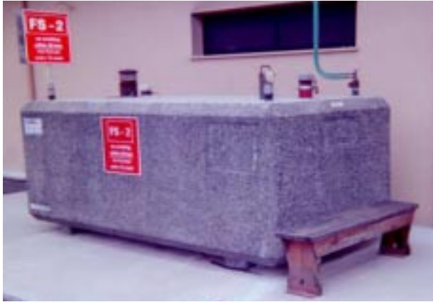
Above Ground Storage Tank
