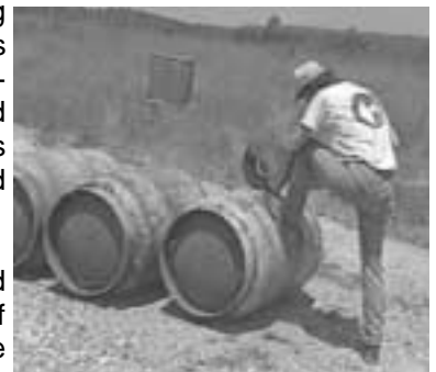
Cylinder decommissioning at the end of the project. Empty/rinsed cylinders were cut in half using a demolition saw
