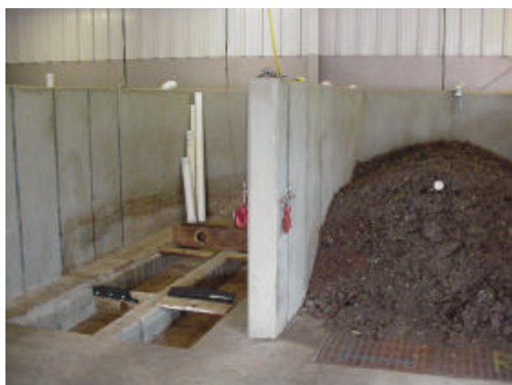
Figure 5. Photograph of two of four compost bins showing the drainage/aeration system. A mixture of wool waste and cotton gin trash is shown in the bin on the right.
