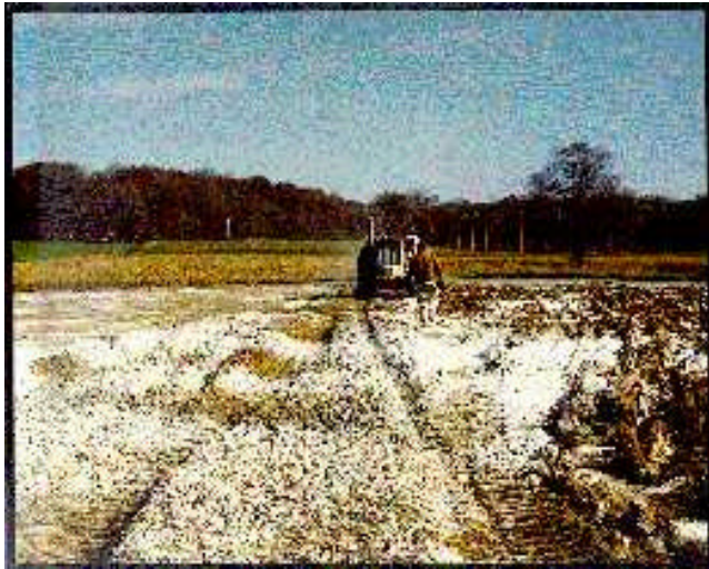
Figure 2. Transition of pad from the ripped soil with lime amendment (right), tilled soil to mix in lime and water (center) and rolled soil to form smooth pad surface (left)
