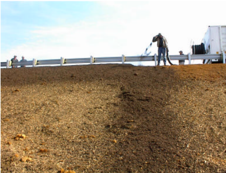
Band-Aid for construction scar
