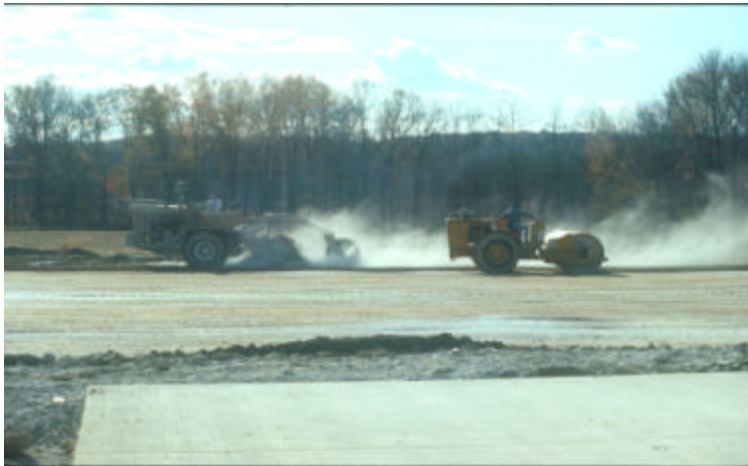
Figure 3. Photo of rototilling and roller equipment working in tandem to form lime stabilized pad. Steam is formed when quick lime and water come into contact.
